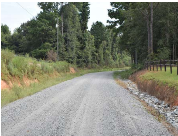
Well maintained unpaved road; wide, grassed, rock lined ditches. Mitchell County Georgia. Photo courtesy of Golden Triangle RCD
