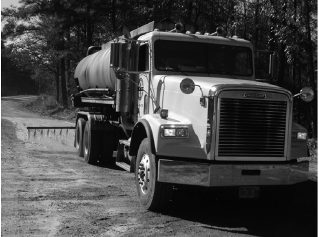
Petroleum emulsion application. Harris County, Georgia Photo: Courtesy of Two Rivers RC&D Council
