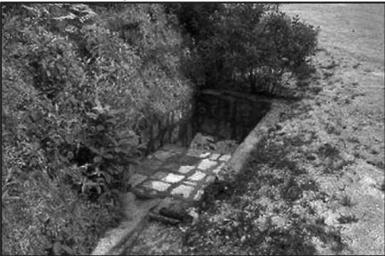
Example of inlet drop box. Source: US Forest Service Low Volume Roads
