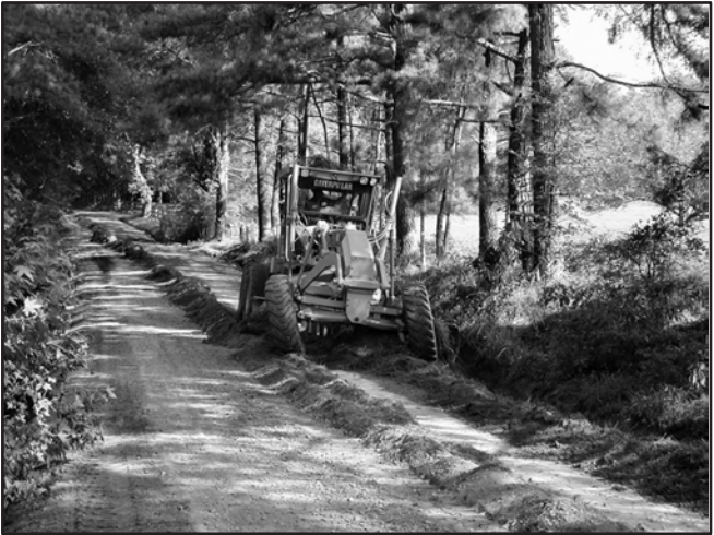
Example of "pulling" ditch and re-establishing crown. Monroe County, Georgia Photo: Courtesy of Two Rivers RC&D Council
