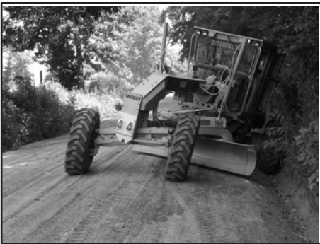
Using wheel for "shaping and tamping" ditch; creates a "roll" or "rounded U" shape ditch. Meriwether County, Georgia Photo: Courtesy of Two Rivers RC&D Council
