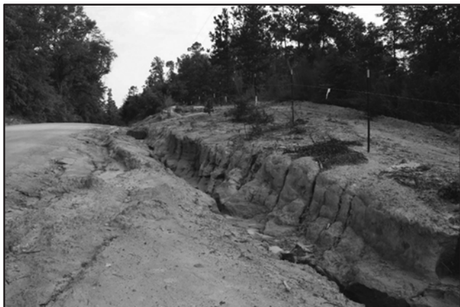
Before Implementation: Eroding road surface, road banks, and ditches
