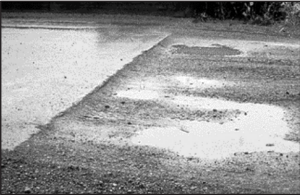
Gravel to pavement problems: potholes.
