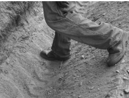
Final shape of roll ditch is a rounded U-shape. Ditch needs to be revegetated. Meriwether County, Georgia
