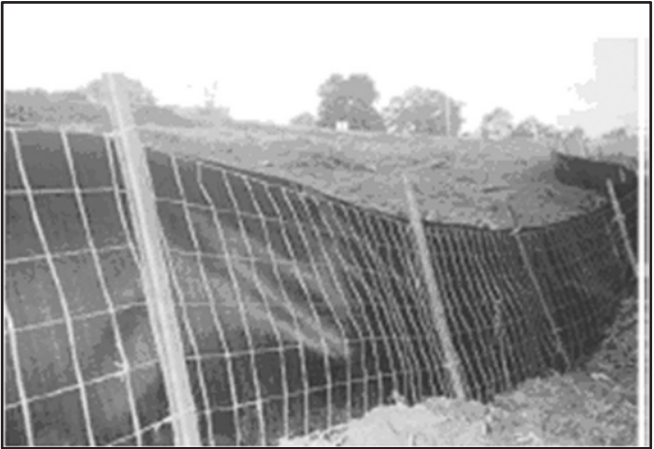
Example of type "C" sediment barrier silt barriers (Sd1-C). Note that the fence is slightly angled into the direction of runoff. Source: Georgia Soil and Water Commission Erosion and Sediment Control Manual
